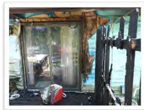
Structure Fire, Norwich Street
