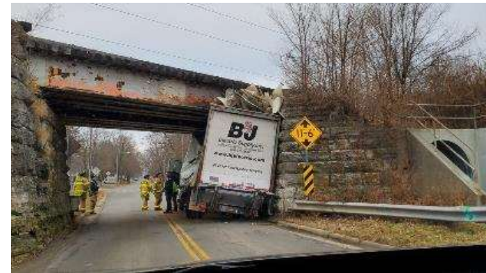
Truck stuck under railroad bridge in Madison, 2019
