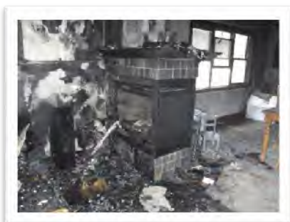
Blazing Star Lane Structure Fire
